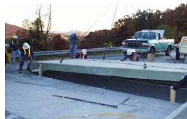
Use of fiber reinforced polymer deck panels for rapid repair of bridge structures.
